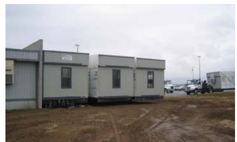
Four new modular building sections await final placement next to the existing facility in mid-September.
